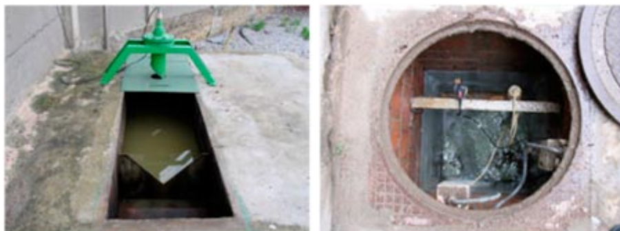
Figura 4.3. Vessadors o canals Parshall .
