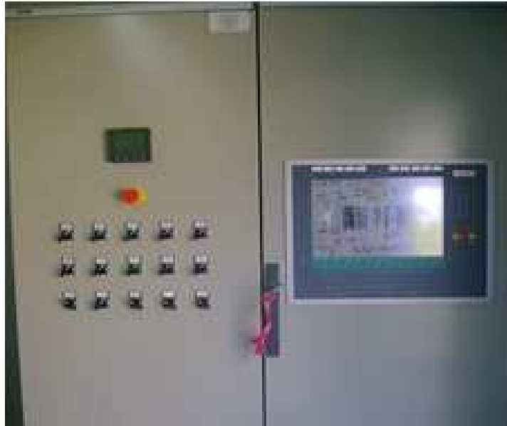
Figura 7. Panell de Control
