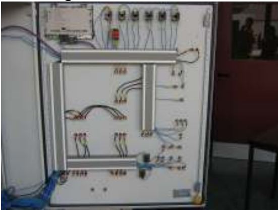
The wiring of the enclosure
