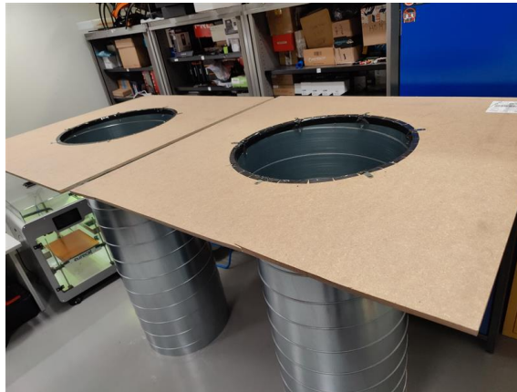
Figure 4.14: The cylindrical tubes installed in the lab at Eurecat Robotics Company
