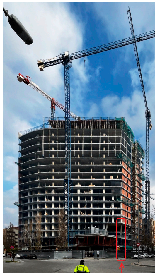
Figure 2. Image of the hotel structure completed in January 2022. You can see the temporary vertical pillar (indicated with a red rectangle), which has not yet been removed.
