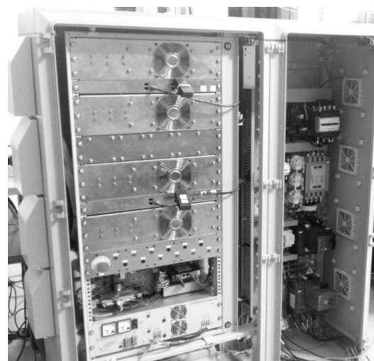
Figure 14. VSVC power converter.
