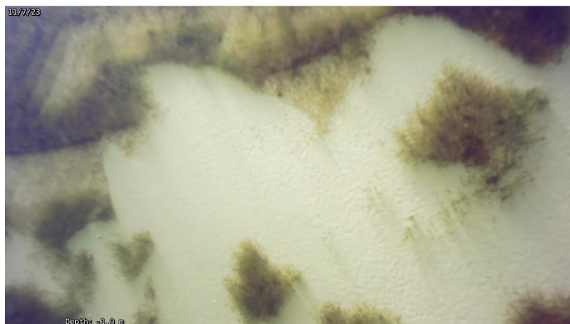
Figure 5.6: The effect of the brush on the Durius structure exposes its surface, enabling an appropriate inspection.
