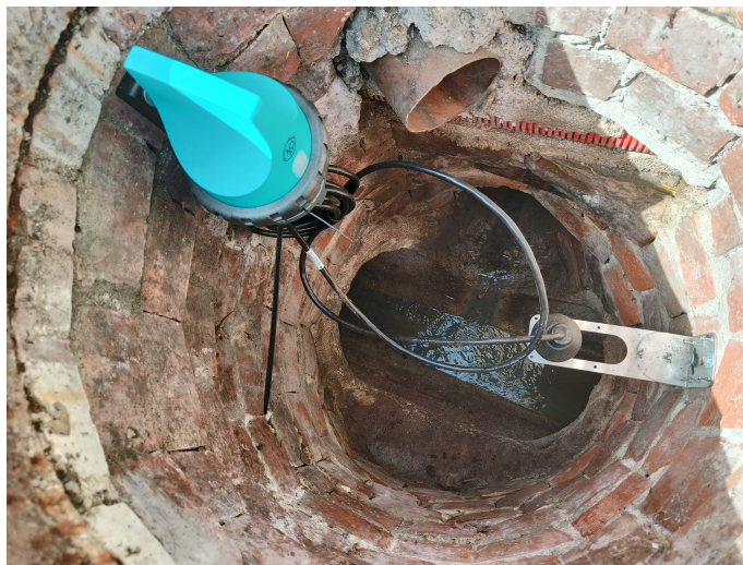
Figure 2.1: Sensor deployment in a wastewater network maintenance hole for flow monitoring purposes. Source: Cicle de l'aigua del Ter.
