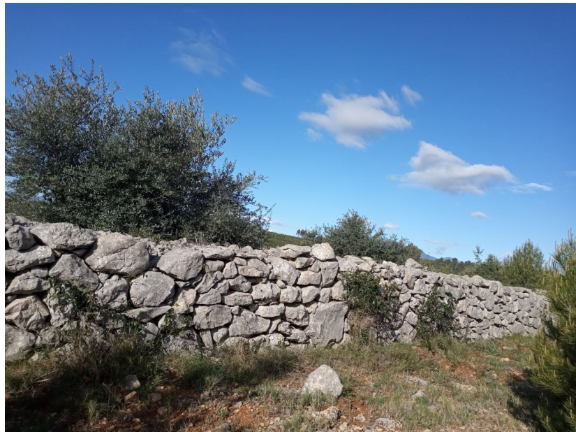
Fig. 1. Photography of a dry stone wall construction in Llers, Catalonia. Own source.
