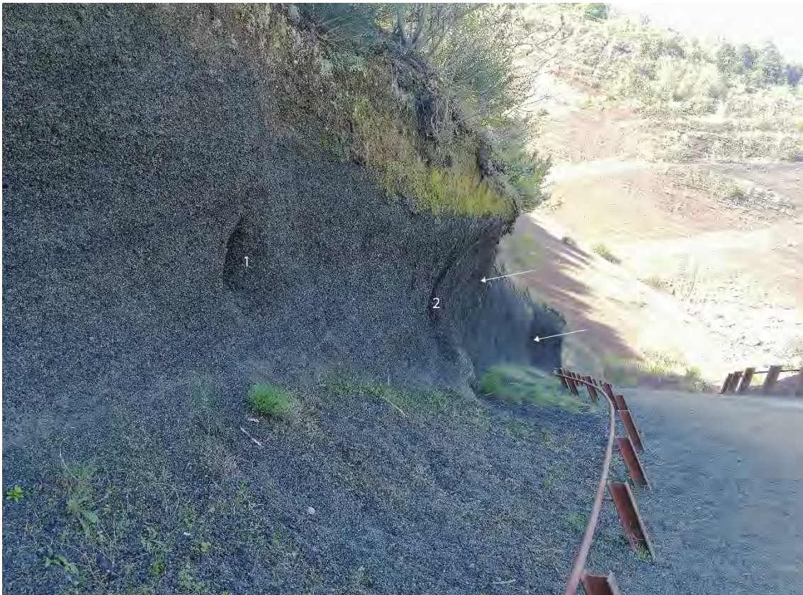
Figure 25. Example of the erosion caused by visitors to the outcrops in the former quarry in Croscat volcano. 1 and 2 are holes that have been dug by hands; the arrows indicate where the wall has collapsed after the continual scratching of the surface of the lapilli by visitors.
