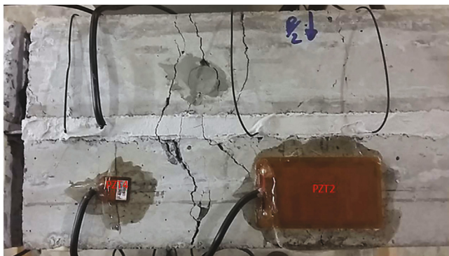
Fig. 4. PZT sensors 2 and 4 on the beam after the damage state 6.
