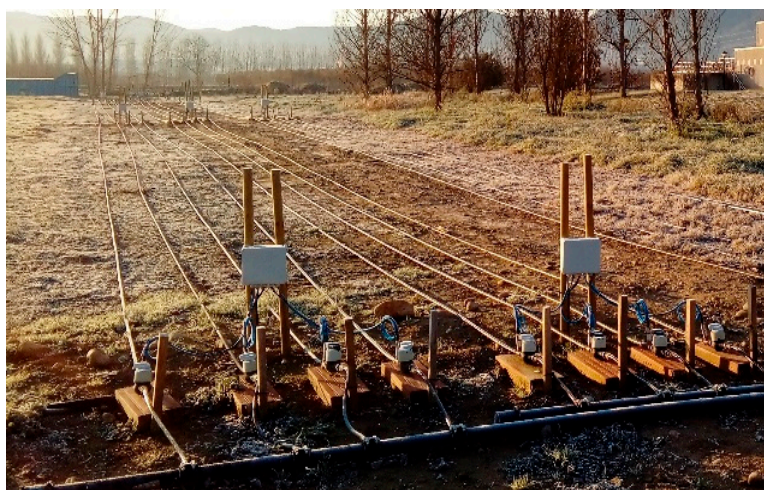
Figure 2. View of the pressure transducers and water meters of the irrigation subunits.
