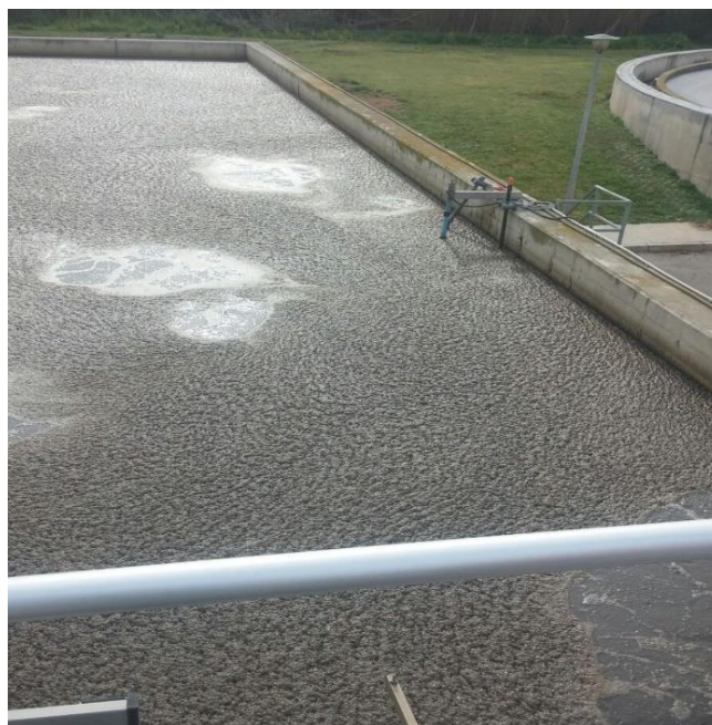
Figure 5. Secondary treatment tank where we sample the sludge.
