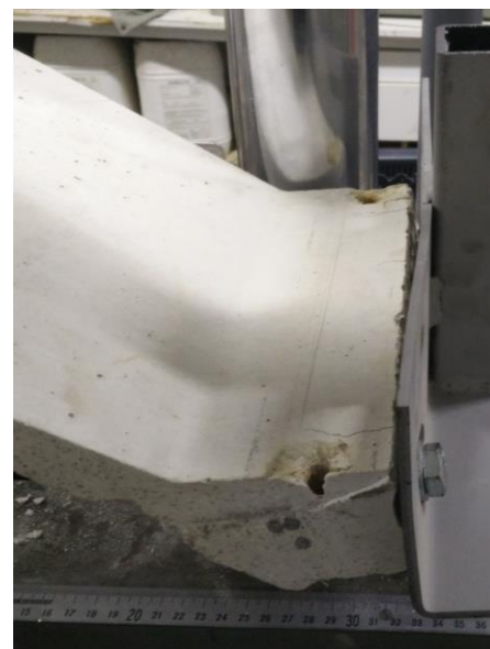
Figure 3: Deformation of the connection (A=12mm)
