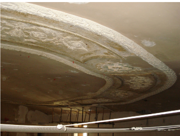
Fig. 2. The damaged lower surface of the historical thin vault of the “Filarmonici” Theatre-hall in Ascoli Piceno (Italy).
