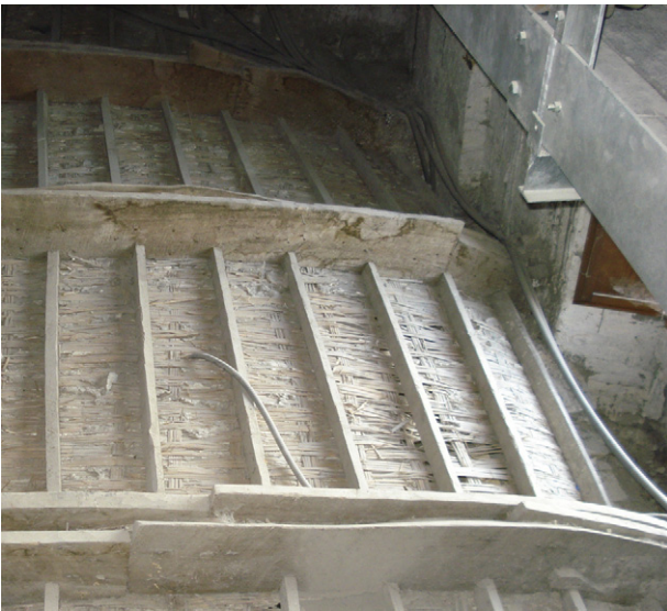
Fig. 1. An example of a thin vault made by timber arches, reeds, and mortar.
