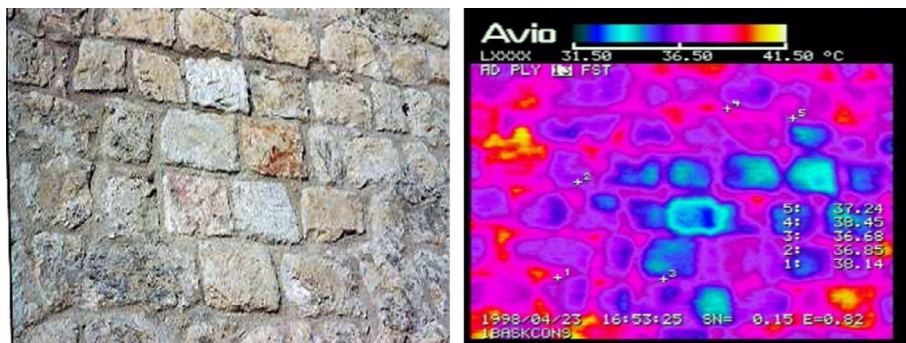
Fig. 2. Left: Fortification masonry facing the National Stadium of Heraklion in Crete; Right: infrared thermograph of the same masonry.
