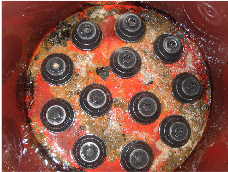
Figure 2. View of nozzle distribution on the perforated plate located at the bottom of the sand bed.
