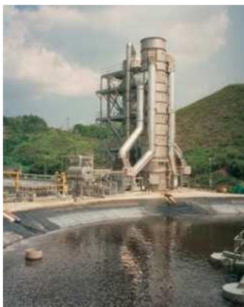
Figure 1.2. View of an ammonia steam stripping plant for the treatment of landfill leachate in the United Kingdom.
