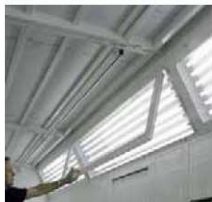
Hinged light fixtures for ease of cleaning and maintenance.
